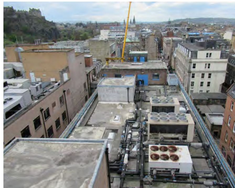
3 – Rose Street roof condition with exposed plant equipment
