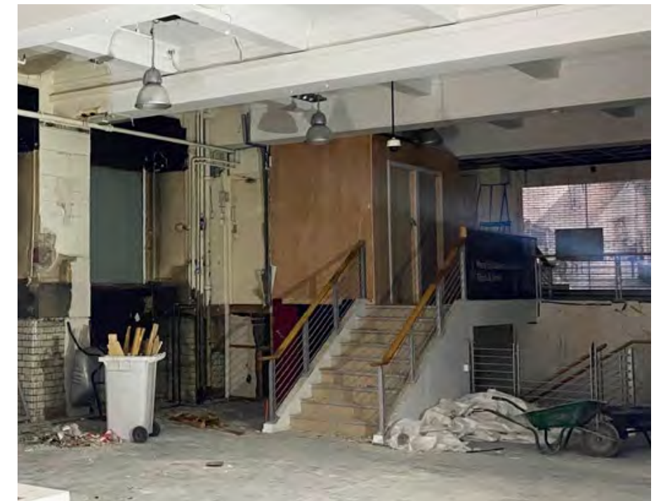
D - 1903 Rose Street internal entrance view with 1200mm level difference
