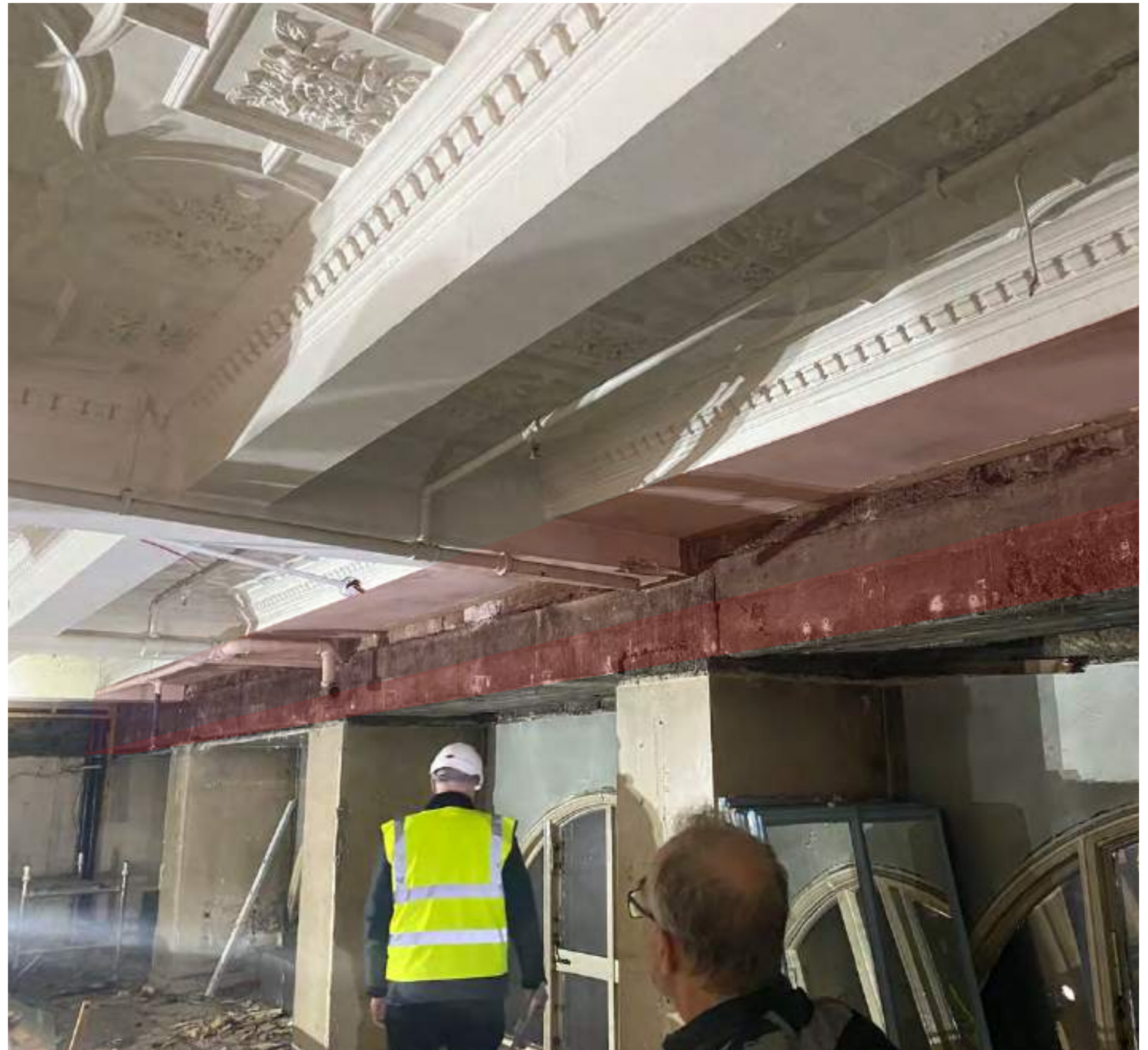
existing condition around mezzanine level facade - a natural break in the decorative ceiling allows local integration of air ducts (highlighted red)
